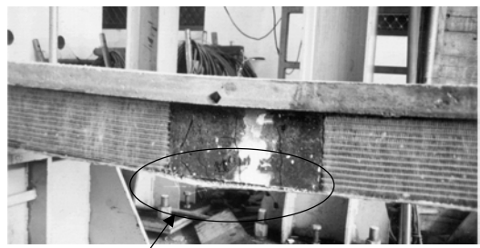
Concrete crack and PGFRP sheet spalling on the bottom
