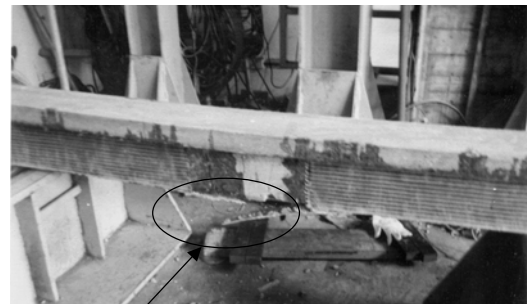
Concrete crack and FRP sheet spalling on the bottom
