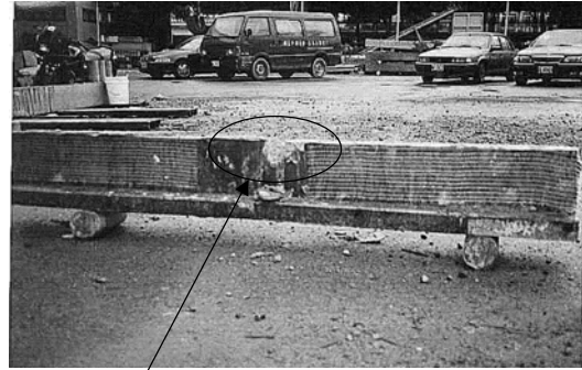
Fig.13 Failure on the top of Beam LFB
