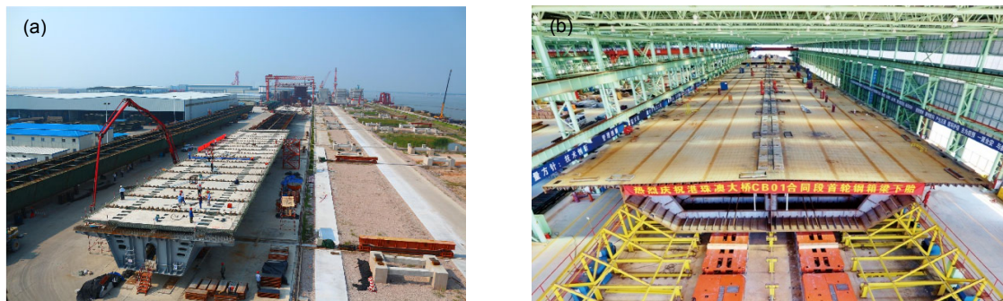
Fig. 3 Superstructure of the bridges on non-navigable waters: (a) 85-m composite girder; (b) 110-m steel box girder
