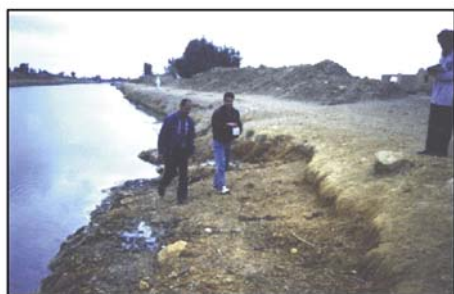
Fig.2 Collapses of the canal bank due to the seepage effluent
