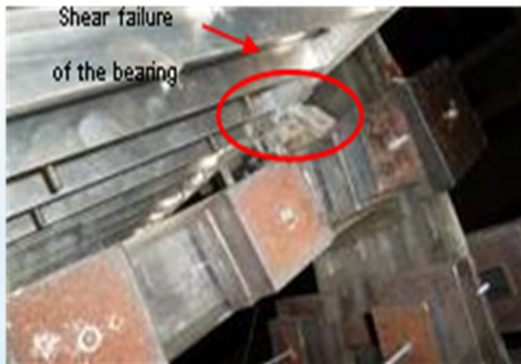
Shear failure of bearing at middle tower
