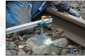
LVDT and accelerometer on sleeper
