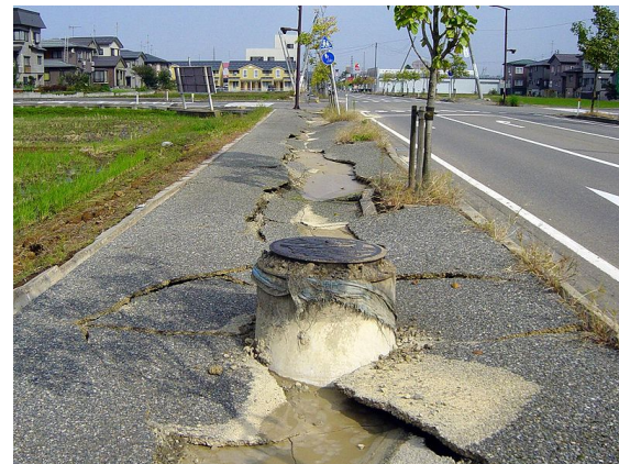
Uplift of buried structures (2004 Chuetsu Earthquake)
