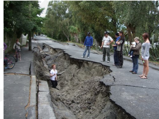
Lateral spreading (2011 Christchurch Earthquake)
