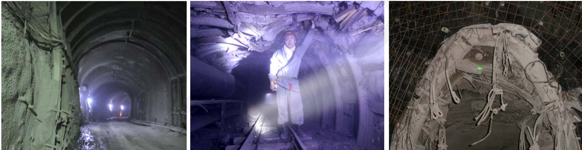
Fig. 1 Arch support failure cases in tunnels
