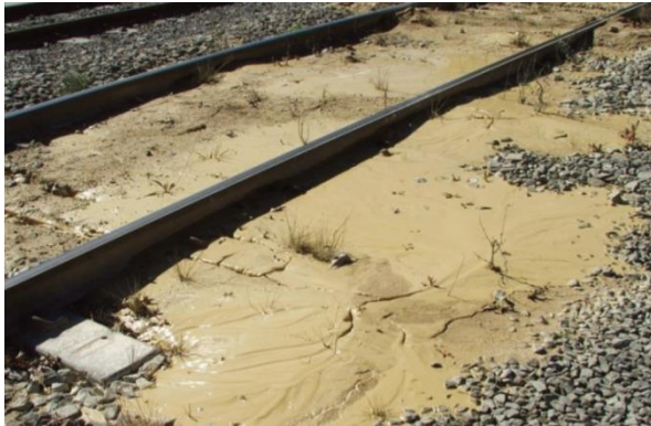
Mud pumping of Ballasted track
