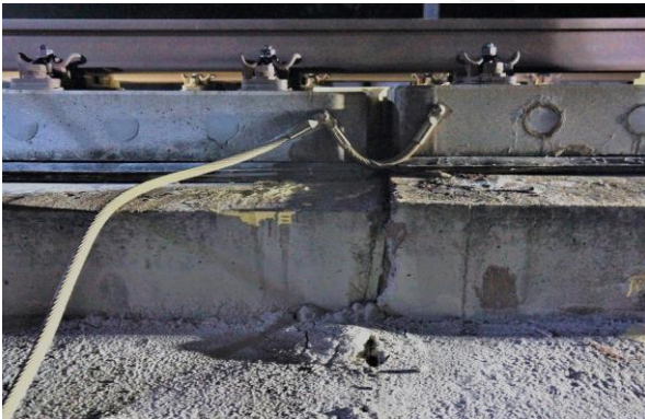
Mud pumping of Ballastless track
