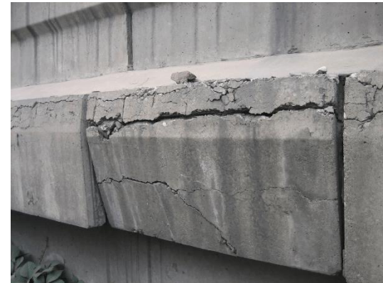
Cracking and degradation
