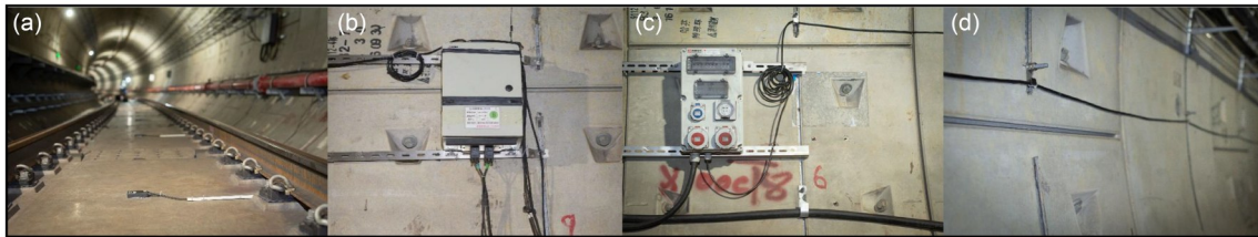
Fig. 10 On-site monitoring system: (a) monitoring module; (b) monitoring terminal; (c) power supply; (d) signal line
