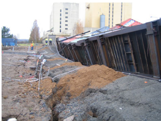
Fig. 12 Full-scale embankment failure loading experiment The loading wagon fallen due to the failure on right and extensive soil instrumentation arrangements on left
